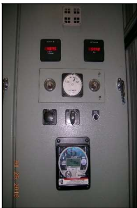
New Control Panels
