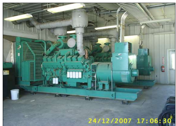
Units 7 & 8 (Unit 7 is in the foreground)
