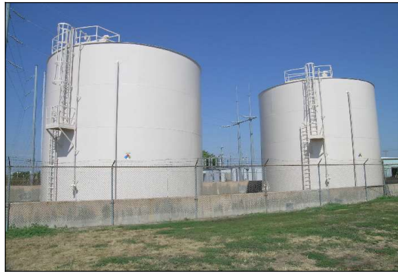
Diesel Storage Tanks
