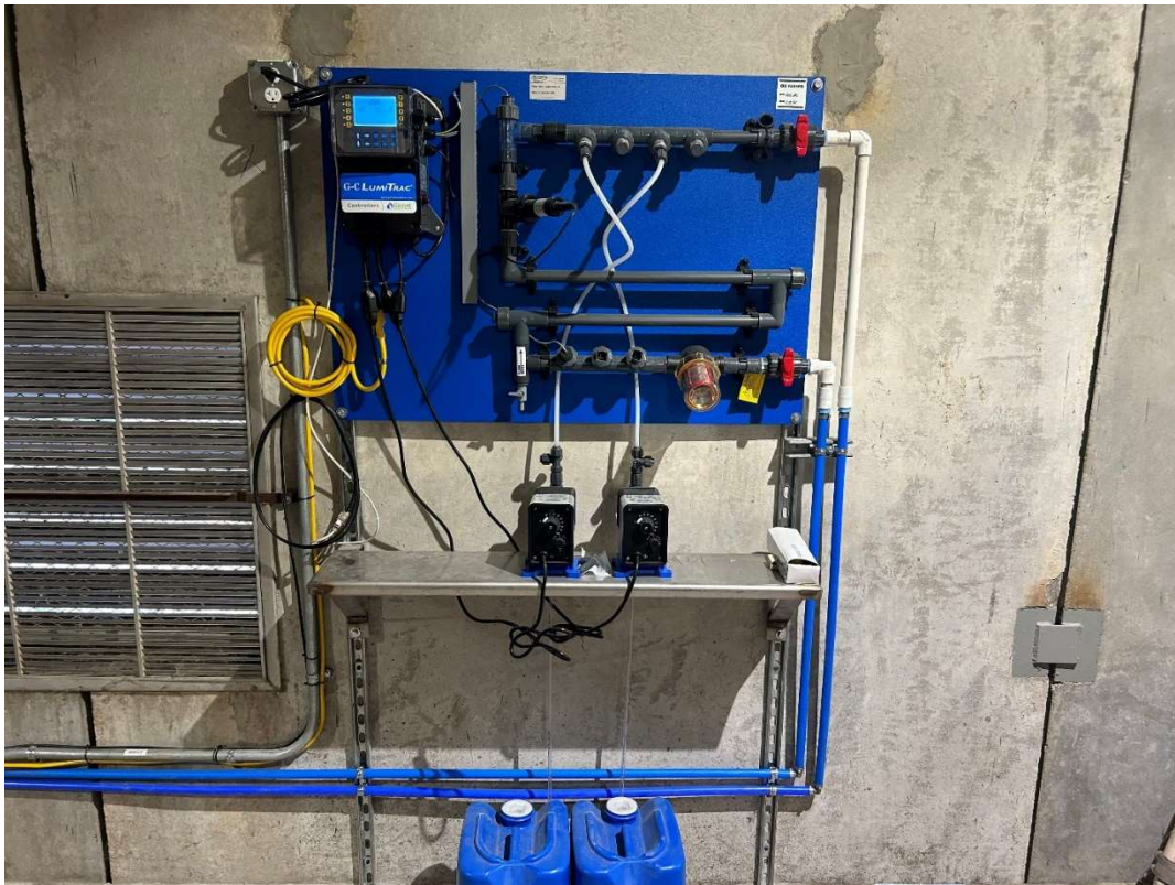
Units 10 & 11 water treatment
