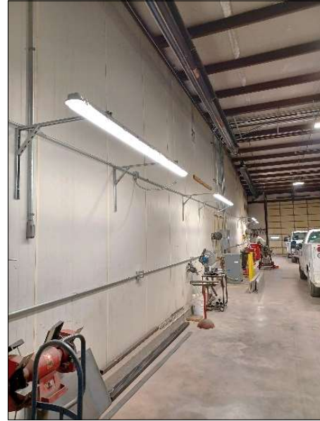
New Task lighting
