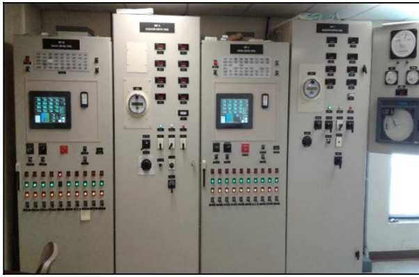
Unit # 10 and #11 Controls
